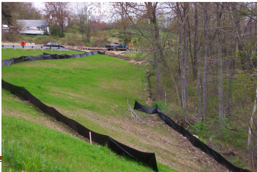
Example of Silt Fence Sedimentation Control
